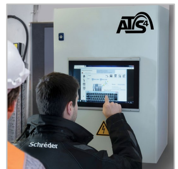
Fully compatible with the latest tunnel lighting control systems, enabling rapid response to incidents and changing conditions inside or outside the tunnel.
